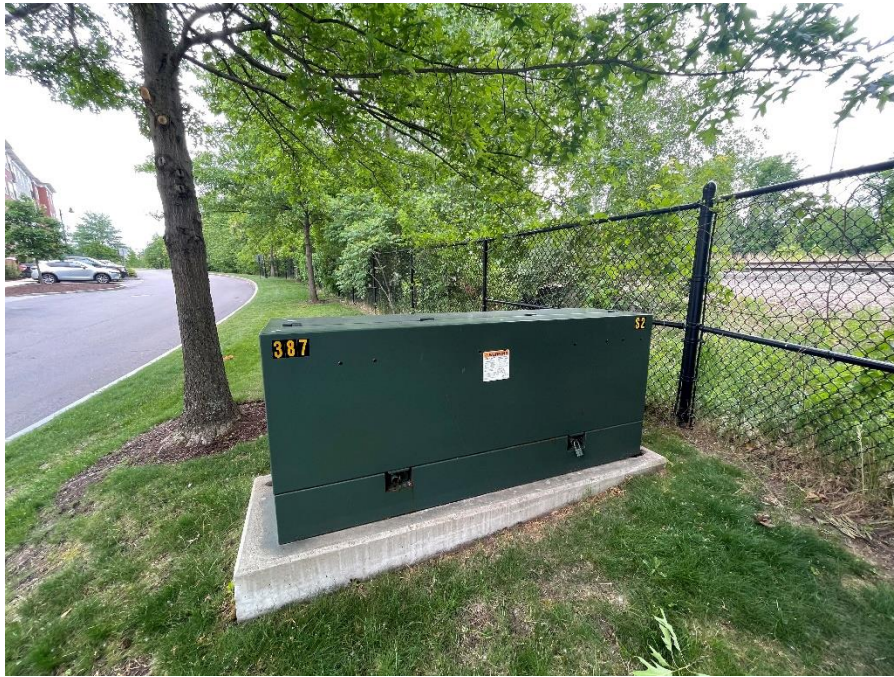
Area F: View of pad-mounted transformer located east along South Commercial Street.
