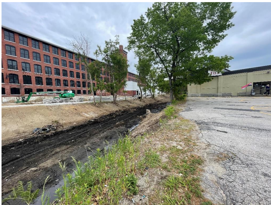
Area C & G: View of the former Electropac/Johnson Shoe facility under construction along the railroad corridor, facing south.
