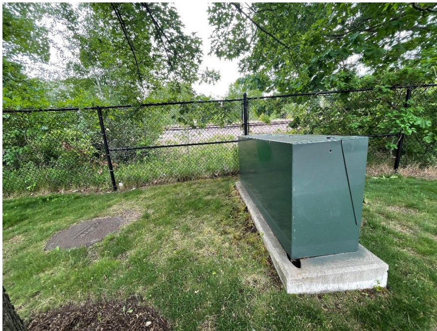
Area F: View of electric manhole associated with transformer observed.
